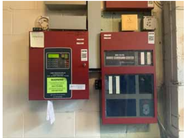
22 - FIRE ALARM PANEL
